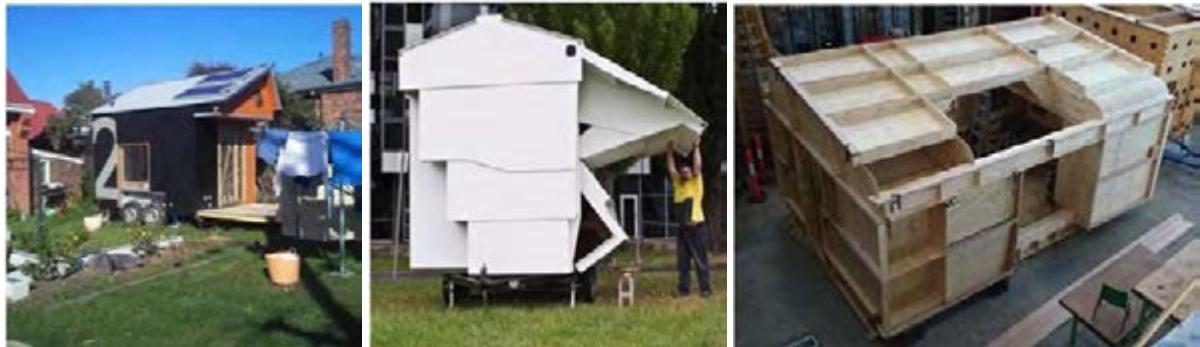
Figure 1. A selection of projects from the LBM digital fabrication research activity (left to right): The Castle2 in backyard setting; The Castle5 – unfolding; Scout-hut prototype).
